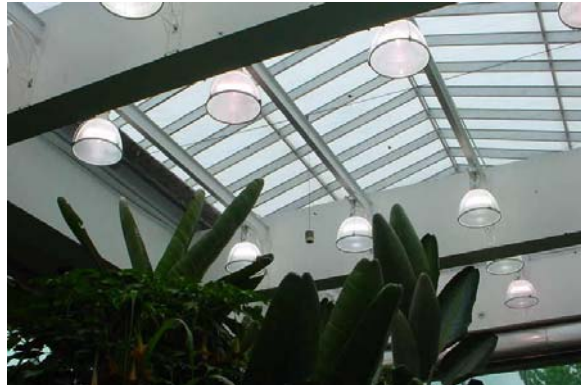
Metal Halide Lights at the Pacific Science Center, Seattle Photo: Hazel Davies
